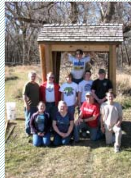
Kiosk erectors showing off a job well done: front, left-right - Angela and Lori Hosford, Dale Bonge and Todd Wynn; back row - Paul and William Hosford, Alec Wynn, Drew Bonge and Curtis Thompson. On top is Miles Wynn, the Eagle Scout kiosk builder. Photo by Amber Wynn.
